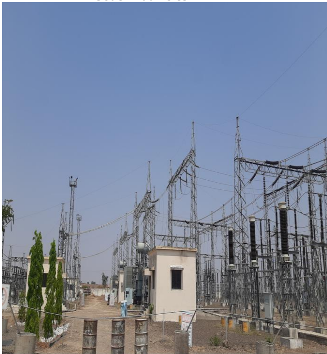
220/33 kv Khanapur PSS
